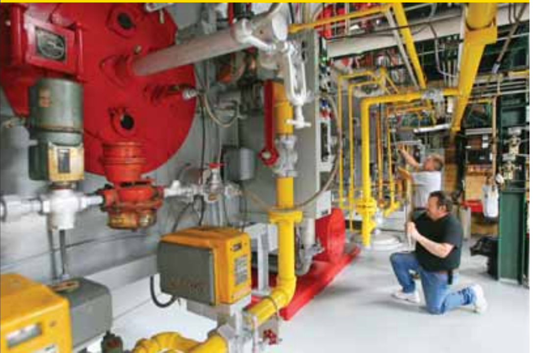
Leroy Staley and Bob Houston, both utility plant operators for Cal U, work on the boilers in the power plant on campus. Cal U's exemplary energy management program was recently highlighted in the PASSHE's 2006-2007 Green Report.
